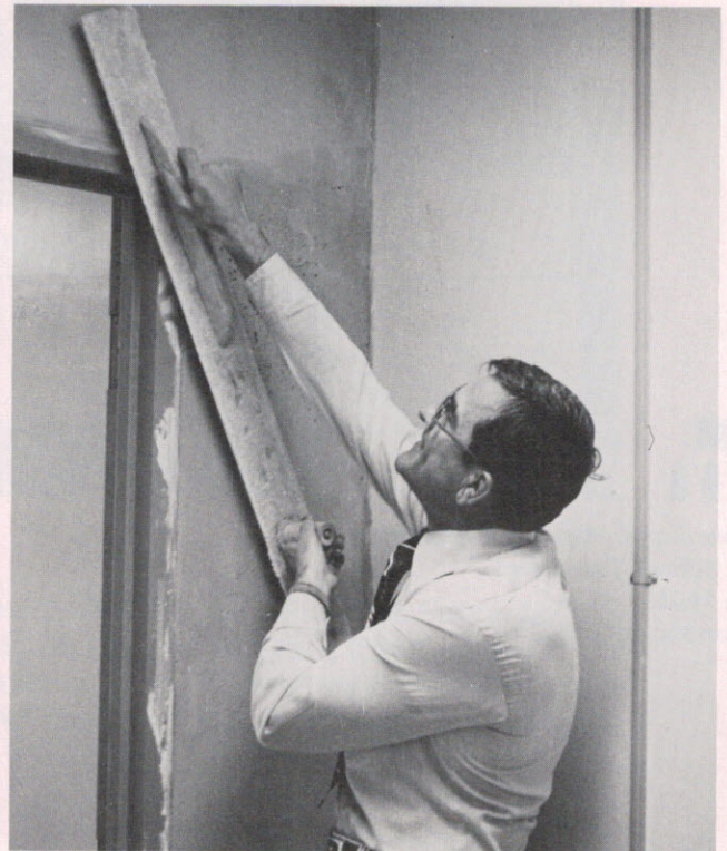
Dean Allen Smith demonstrates his skills (?) plastering a new wall as Tate Hall is remodeled to gain badly needed space.
